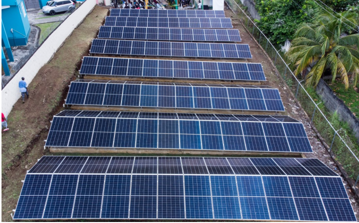
KCCU's Solar farm at Kingstown Park
